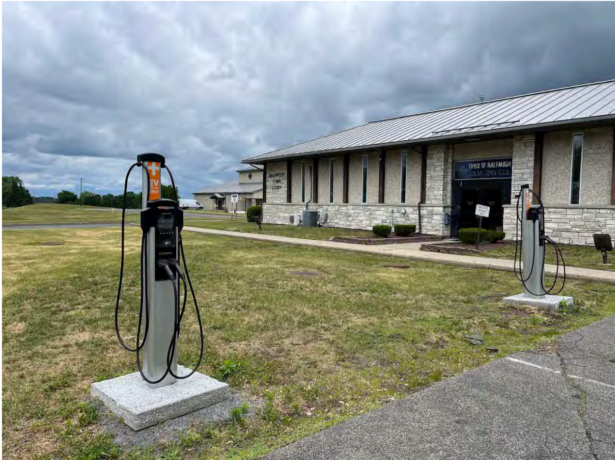
Photo of EV Chargers at Halfmoon Town Court
